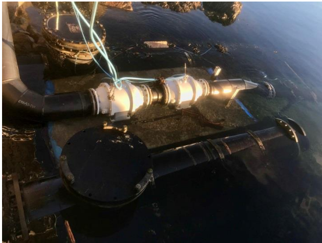
Two pumps in series
